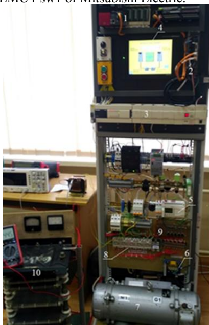
Fig. 1. View of the control part of the laboratory installation: 1 – PLC series IQ-R; 2 – Servodrive Amplifier MR-4J; 3 – PLC series FX3U64M; 4 – HMI GOT-1575; 5 – PLC Alpha2; 6 – Speed Sensor; 7 – Asynchronous Motor – DC Generator Aggregate; 8 – Solid State Relay (switches); 9 – Manual Setting Load Range; 10 – DC Generator Load Simulator (6 stages of load resistor)
