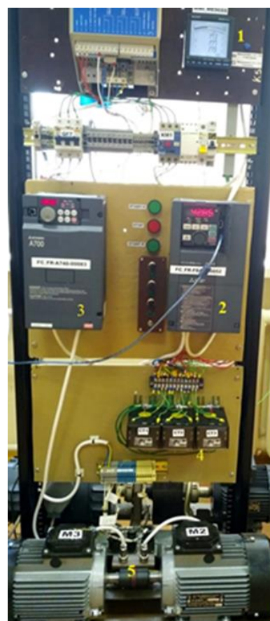
Fig. 2. Frequency converters with asynchronous motors: 1 – Electronic Multi-measuring Device ME96SSRA-MB; 2 – Inverter FR-F840-E2; 3 – Inverter FR-A740; 4 – Current Transformers (output side of FC); 5 – Two Asynchronous Machines Aggregate (1.5 kW)
